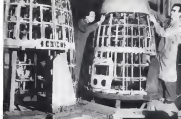
COWLING jobs are being polished over attachment points on forward portion of semi-monocoque structure. Thin ring mounts against double wing to wing post, shape appears heavy enough to carry some engine load.
